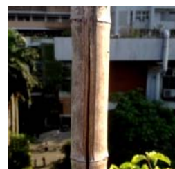
Figure 11. Cracks on bamboo specimen surface 图 11. 竹竿试体表面裂痕
