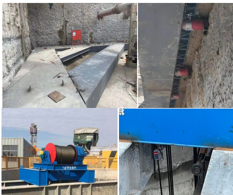
Figure 3. Schematic diagram of sliding fast pre-support system module for deep foundation pit
