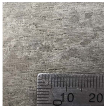
Figure 4. Crack zone morphology 图 4. 裂纹区形貌
