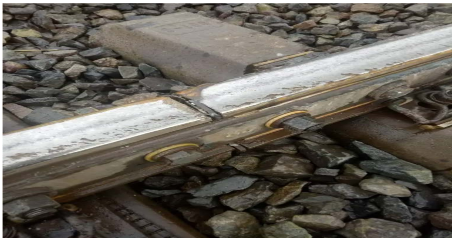
Figure 3. Rail joint damage
