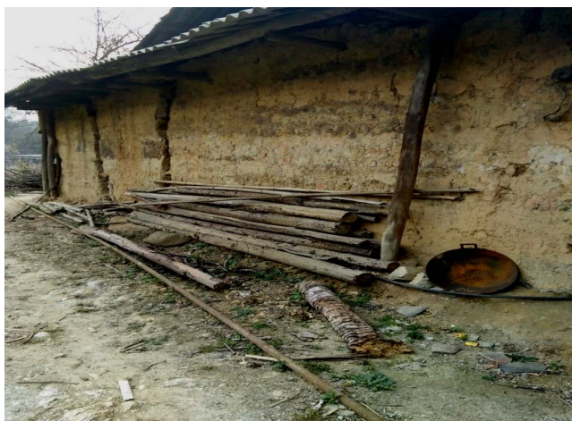
Figure 2. Foundation settlement and building tilt 图 2. 地基沉降 房屋倾斜
