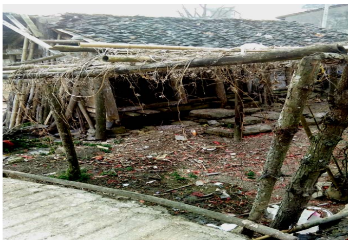
Figure 5. Roof caved and ground subsidence
