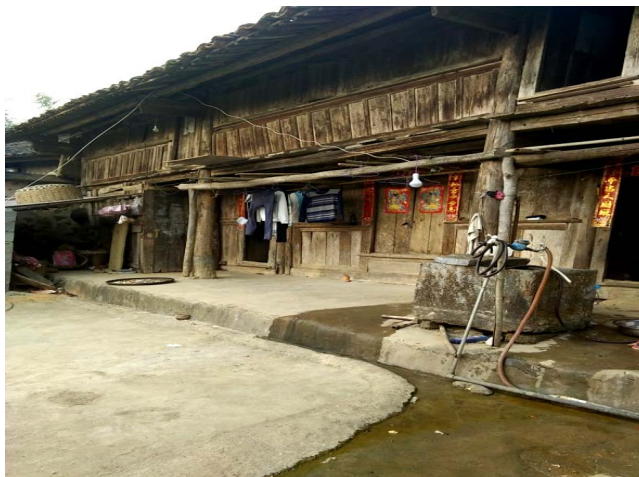
Figure 3. Building tilt, domestic sewage discharged everywhere 图 3. 房屋倾斜、生活污水随处排放
