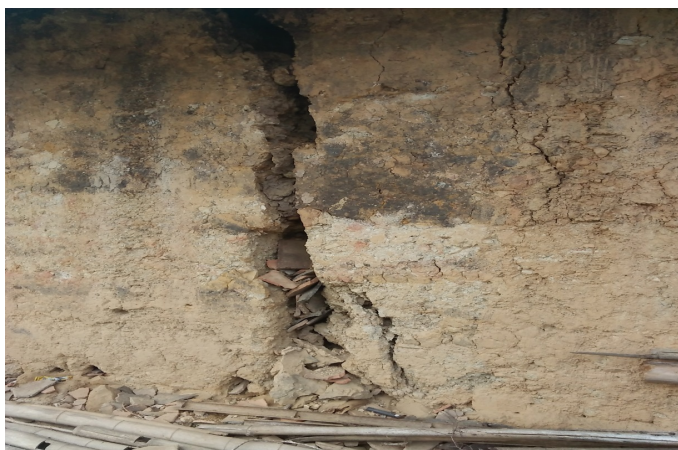
Figure 4. The crack of buildings
