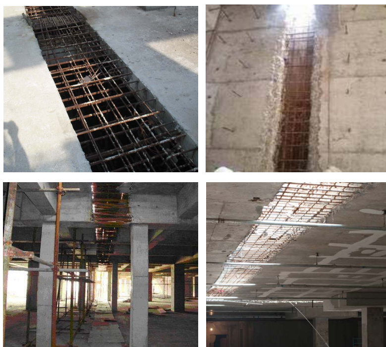
Figure 1. Steel bars across through the post-casting band in reinforced concrete structures 图 1. 横穿混凝土后浇带的结构配筋
