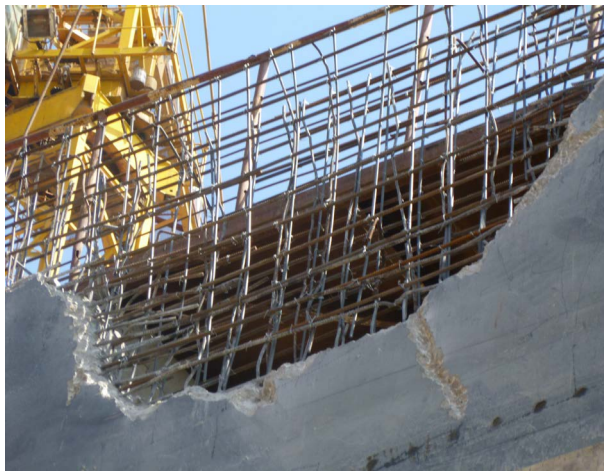
Figure 7. Reinforcing rebar mesh at damaged spots
