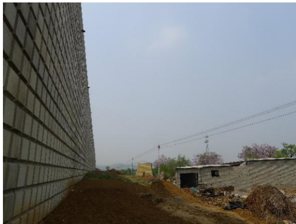
Figure 1. Lateral displacement of the wall
