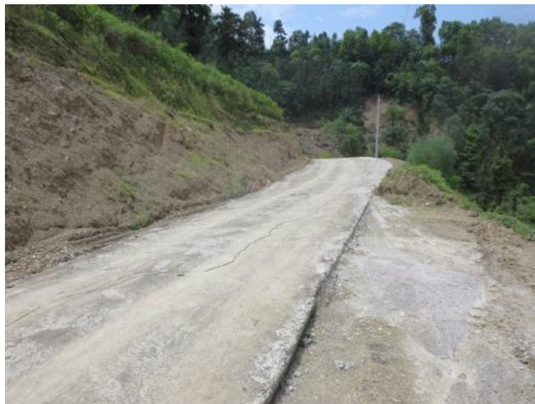
Figure 2. Construction of pavement and subgrade excavation in front of landslide 图 2. 滑坡前缘施工便道及路基开挖
