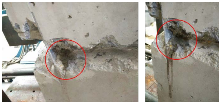
Figure 4. The water seepage of component with traditional steel plate 图 4. 传统止水钢板试样接缝渗水
