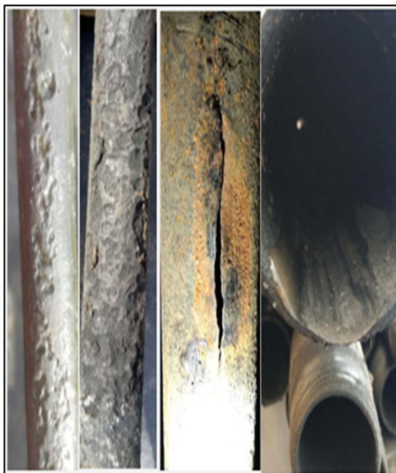
Figure 2. Eccentric wear and corrosion of oil pipe rod during operation inspection
