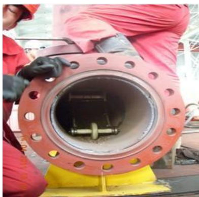
Figure 7. Lower down test of iron scrap recovery device 图 7. 铁屑回收装置下放试验
