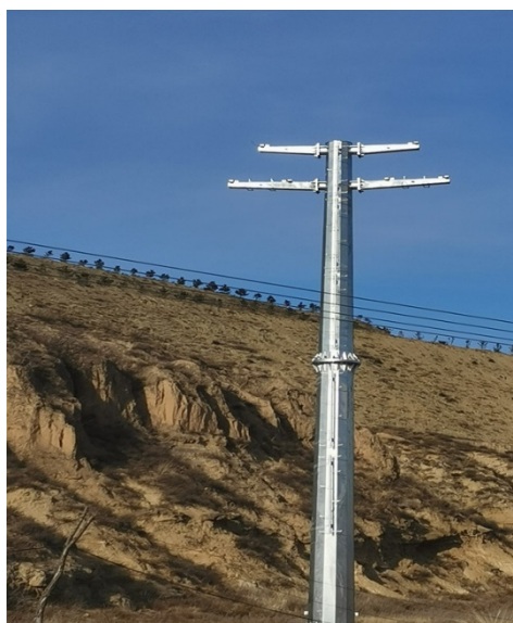
Figure 1. Transmission towers with cantilever cross-arms
