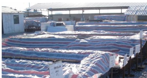
Figure 2. Striped cloth protection and overhead material 图 2. 材料架空并用彩条布进行防护
