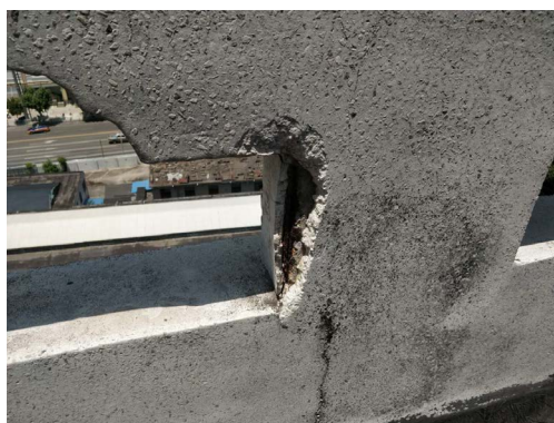
Figure 5. Top floor railing column broken, exposed tendons
