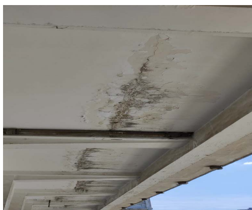
Figure 4. Water seepage in the roof of the 8th floor corridor
