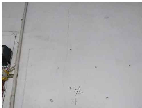
Figure 3. Cracks in the decorative layer of the wall of the 8th floor 4-5/G axis
