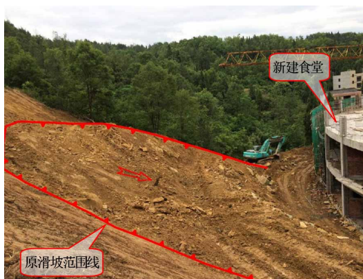
Figure 3. The status quo after slope cutting in north slope section of the site
