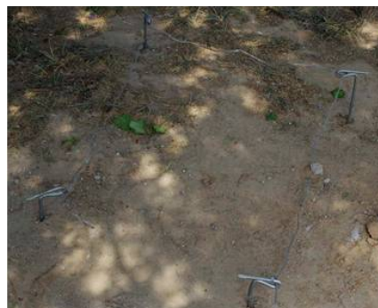
Figure 2. the grounding body device 图 2. 接地体实物图
