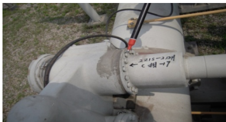
Figure 2. Leakage of grounding switch 图 2. 漏气接地开关
