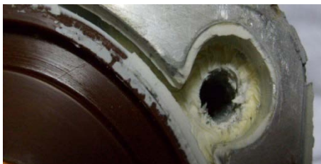
Figure 1. Leakage of ground terminal 图1. 漏气接地端子
