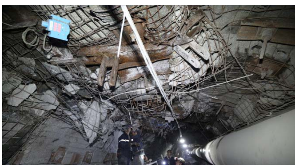
Figure 2. The figure of roadway roof failure 图 2. 巷道顶板破坏示意图
