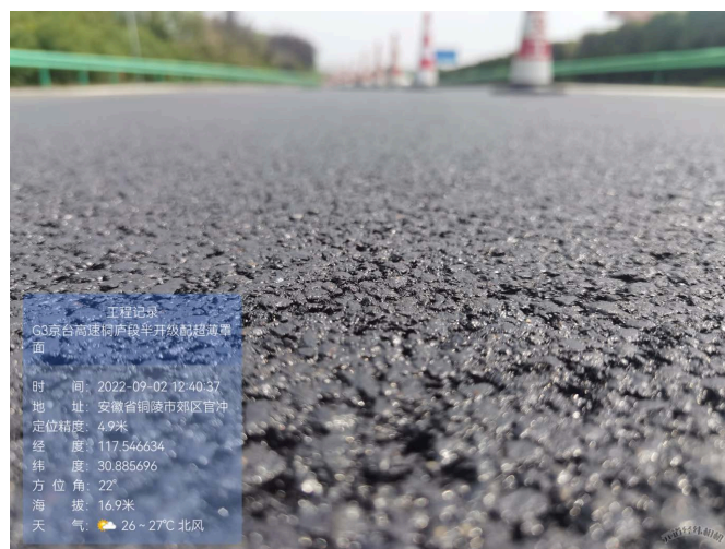
Figure 6. Ultra-thin overlay pavement of high viscosity and elasticity modified asphalt 图 6. 高黏高弹改性沥青超薄罩面施工效果图
