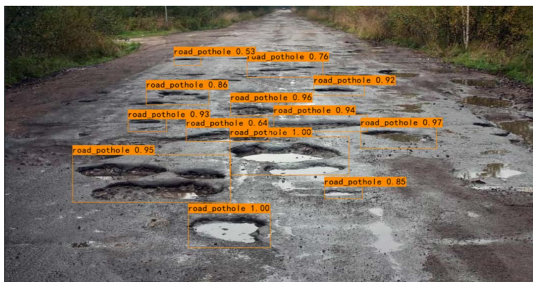
Figure 7. The effect of road pothole detection
