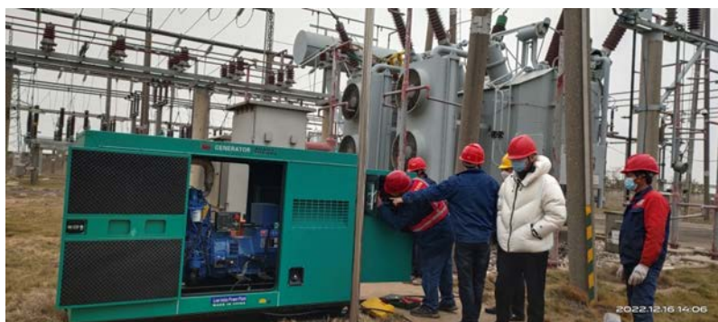
Figure 7. 220 kV Substation #2 main transformer air cooling system uninterruptible power supply reconstruction construction site drawing
