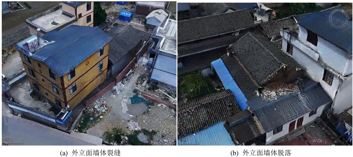
Figure 9. Buildings with obvious damage to the façade but intact roof shape 图 9. 建筑物外立面损毁明显但屋顶形态完好
