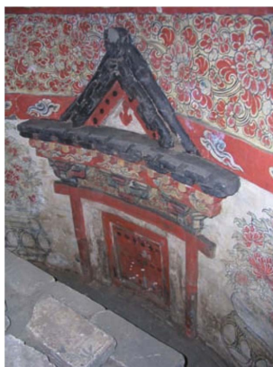
Figure 6. Brick painted false door on rear wall of rear room 图 6. 后室后壁砖雕彩绘假门
