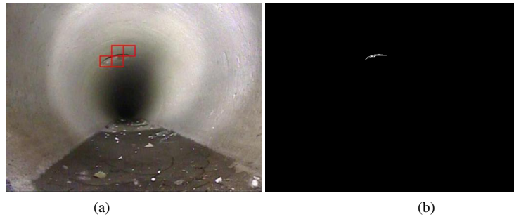
Figure 5. Pipeline image with fracture, (ii) group (a) fracture recognition result marking map; (b) binary chart of fracture recognition result
