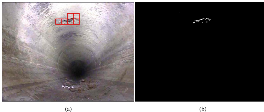
Figure 4. Pipeline image with fracture, (i) group (a) fracture recognition result marking map; (b) binary chart of fracture recognition result
