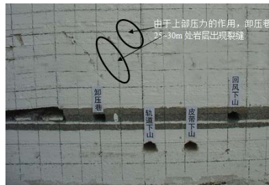
Figure 7. Crack at the top of pressure relief roadway
