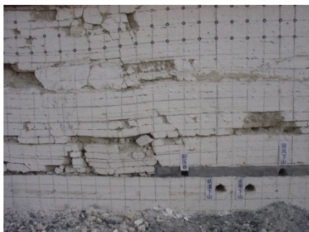
Figure 9. Rock failure around pressure relief roadway
