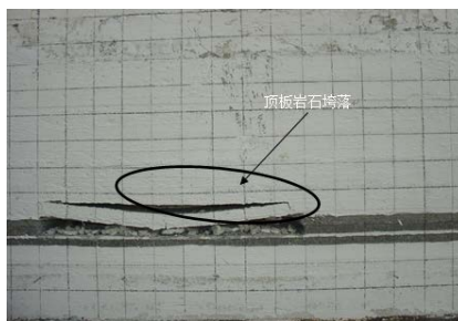
Figure 4. Collapse of roof rock 图 4. 顶板岩石垮落
