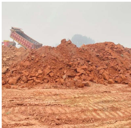
Figure 1. Photos of backfill construction in the test compaction area 图 1. 试夯区回填施工照片
