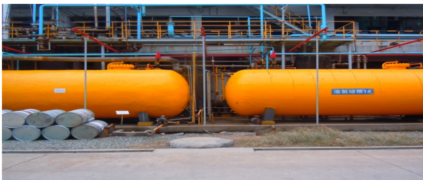
Figure 1. The large tank of liquid ammonia in outdoor 图 1. 室外液氨大槽
