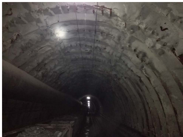
Figure 6. The effect of western third transport stone gate support 图 6. 西三轨道石门支护效果
