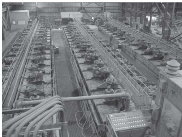
Figure 1. Existing flotation system before renovation
