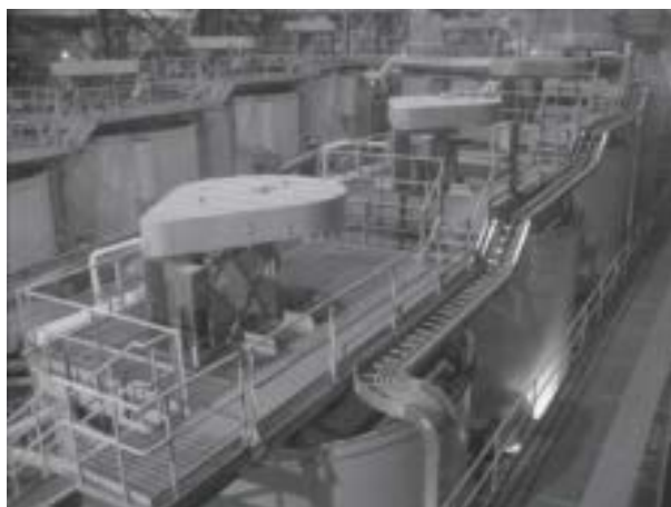
Figure 7. The third stage completed the new flotation cell system operation
