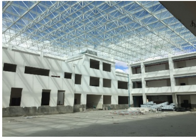
Figure 3. Field photo of the atrium attached sunspace 图 3. 中庭附加阳光间现场照片
