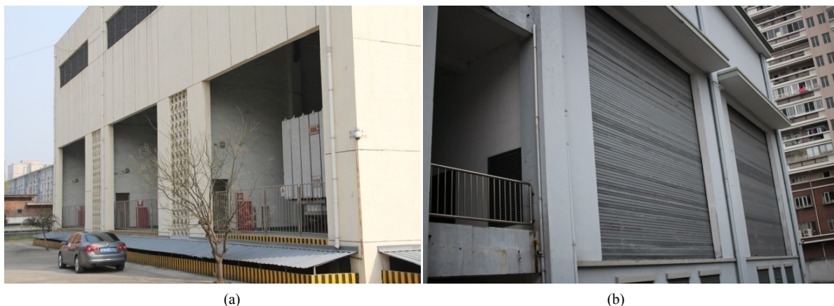
Figure 1. Structure of main transformer door: (a) Open structure; (b) Simple door (rolling door) construction 图 1. 主变室大门结构形式: (a) 敞开结构; (b) 简易门(卷帘门)结构
