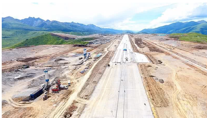
Figure 1. Engineering features of ganzi airport in construction 图 1. 建设阶段的甘孜机场工程特征
