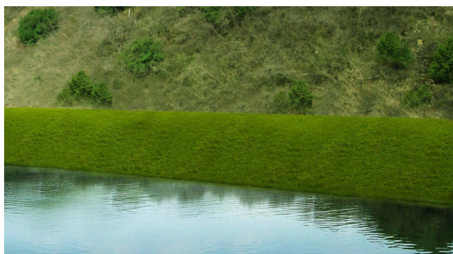
Figure 11. Control effect picture of fluctuation area—lateral vegetation restoration 图 11. 涨落区防治效果图——侧面植被恢复效果
