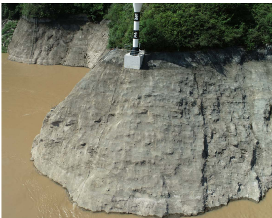
Figure 2. Overview of Dulong (No.1) treatment Project in Wuxia Section 图 2. 巫峡段独龙 1 号治理工程全貌
