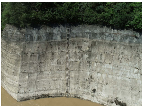
Figure 1. Overview of Maocaopo (No.4) treatment Project in Wuxia Section 图 1. 巫峡段茅草坡 4 号治理工程全貌
