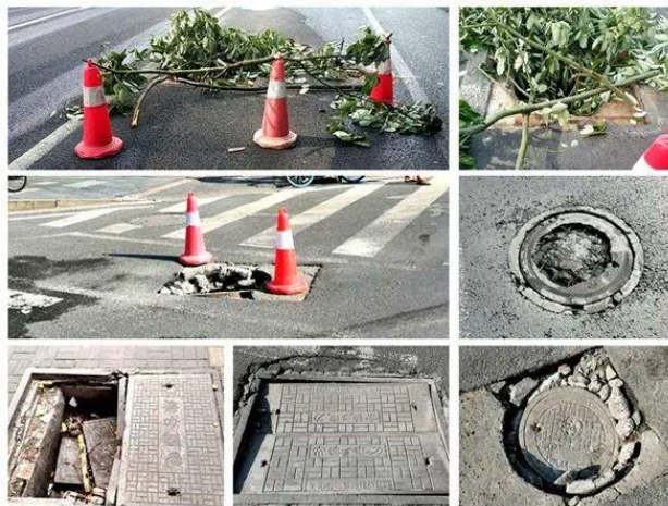
Figure 5. Manhole cover is broken 图 5. 井盖破损 ⑤
