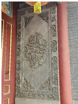
Figure 18. Center wall of the right corridor of No. 129 Lishi Hutong 图 18. 礼士胡同 129 号院右廊心墙 ®
