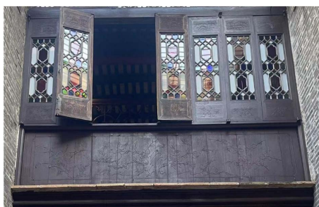
Figure 20. Lu family mansion partition door type window 图 20. 卢家大屋隔扇门式窗 ②
