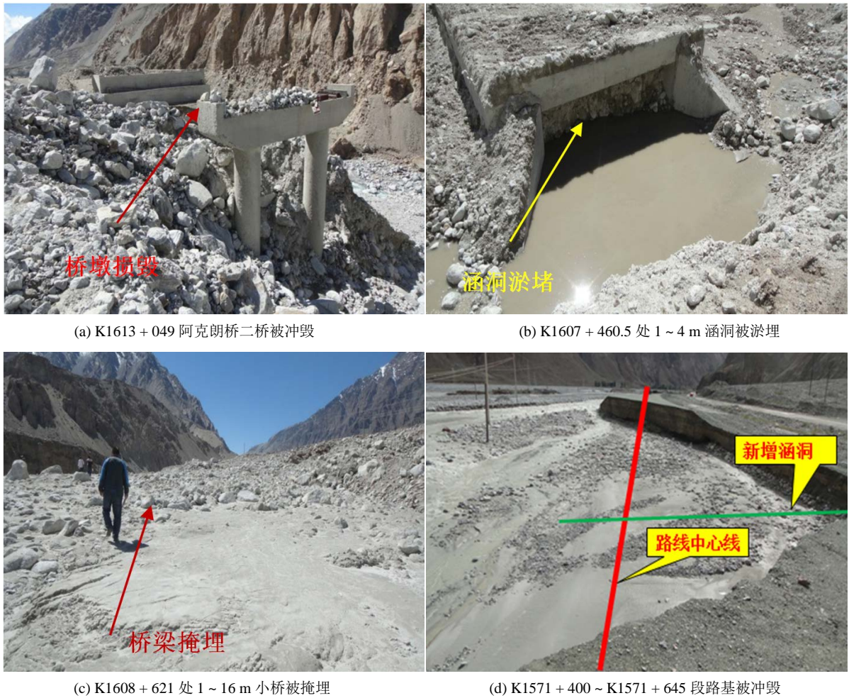
Figure 5. The bridges and culverts are washed way and buried by debris flow 图 5. 公路桥涵被泥石流冲毁淤埋
