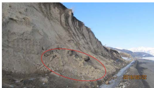
Figure 7. Collapsed in K110+460+K110+520
