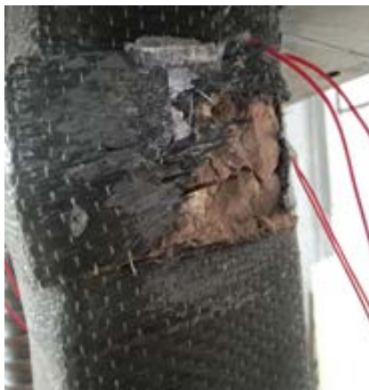
Figure 2. Failure modes of the specimen 图 2. 加固试件破坏形态
