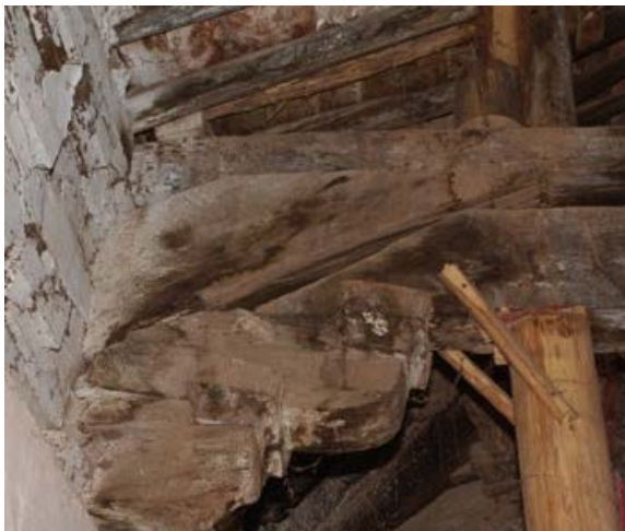
Figure 3. Pulling tenon failure 图 3. 拔榫破坏
