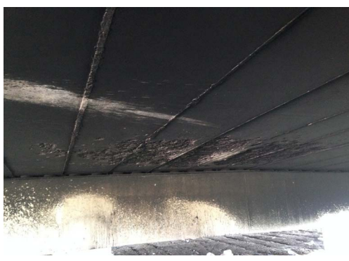
Figure 2. The fired area in the bottom of slab 图 2. 桥梁底部受火区域
