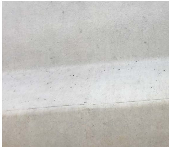
Figure 9. 9# beam's appearance quality 图 9. 9#梁体外观情况
