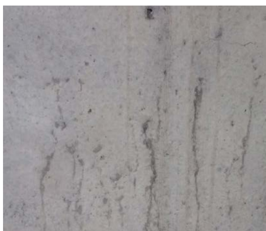
Figure 11. 10# beam's appearance quality 图 11. 10#梁体外观情况
