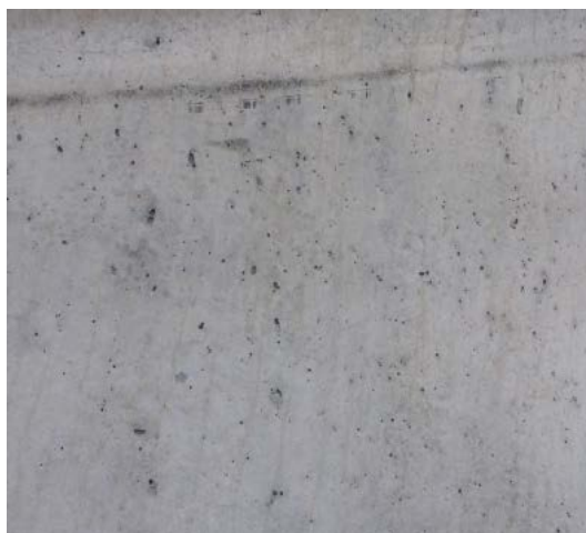
Figure 10. 9# beam's appearance quality 图 10. 9#梁体外观情况
