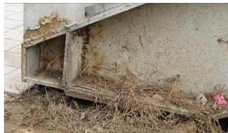
Figure 12. Corrosion of steel plate on landing stairway
