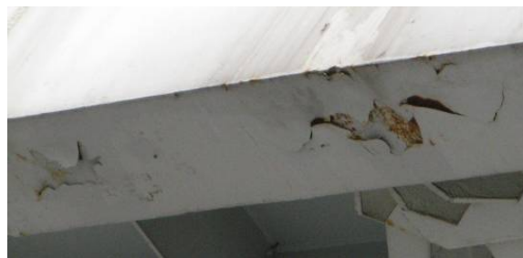
Figure 14. Large area of steel plate rust and paint peeling
