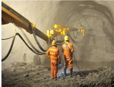
Figure 6. Wet spraying machine hand shotcrete operation 图 6. 湿喷机械手喷混凝土作业
