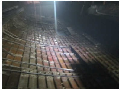
Figure 7. Arc location of inverted arch
