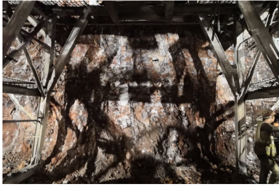
Figure 5. Geological condition of the face of the entrance of Abaisi right Tunnel
