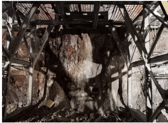
Figure 2. Geological condition of the face of the entrance of Abaisi left Tunnel
