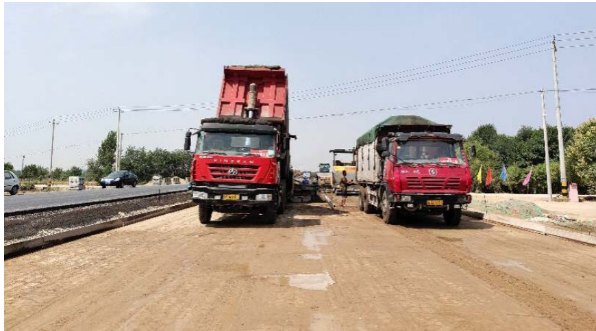
Figure 1. Site construction drawing of cement stabilized macadam base 图 1. 水泥稳定碎石基层双层连铺施工图
