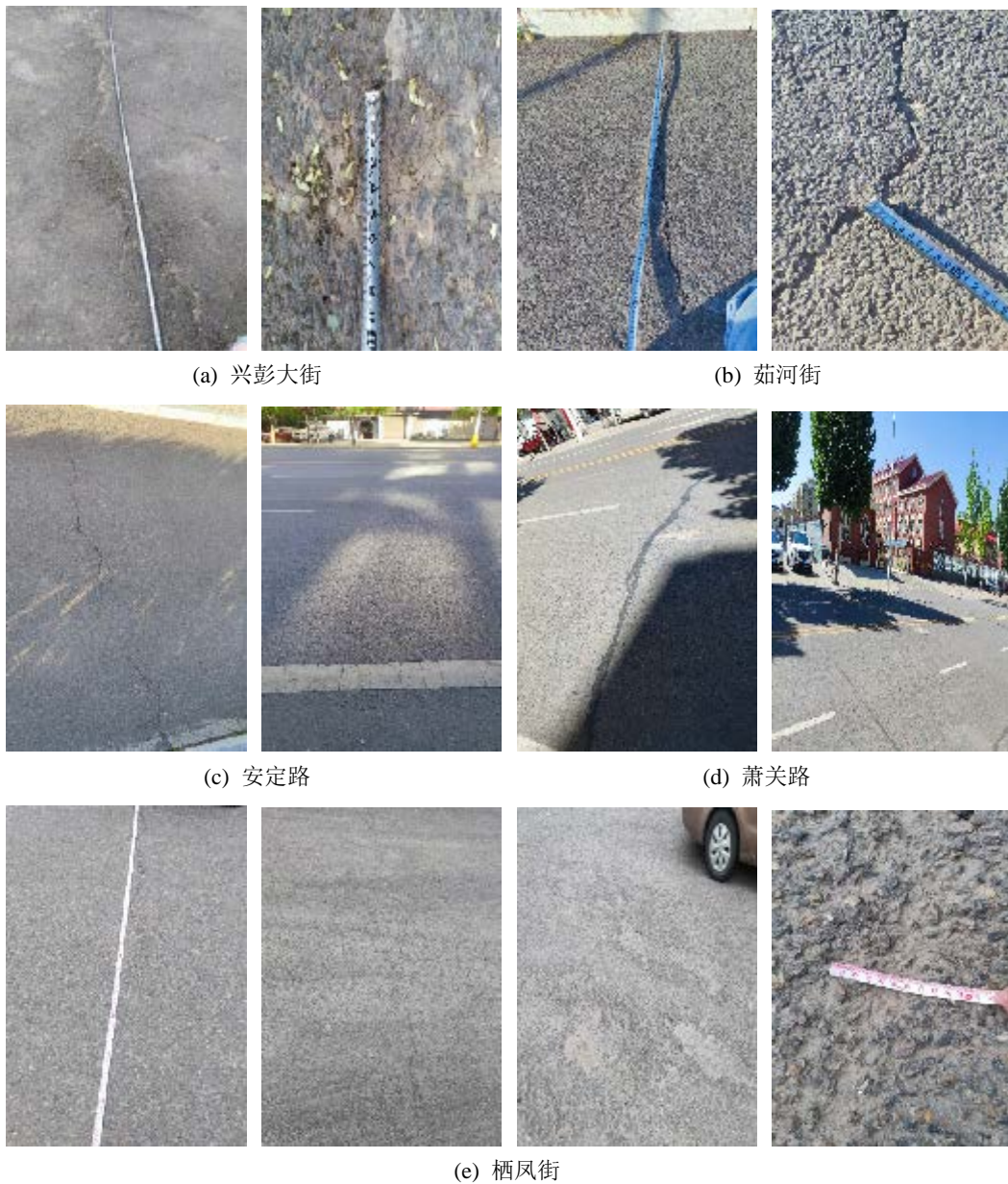
Figure 3. Typical section of pavement damage in Guyuan 图 3. 固原地区典型路段病害情况
