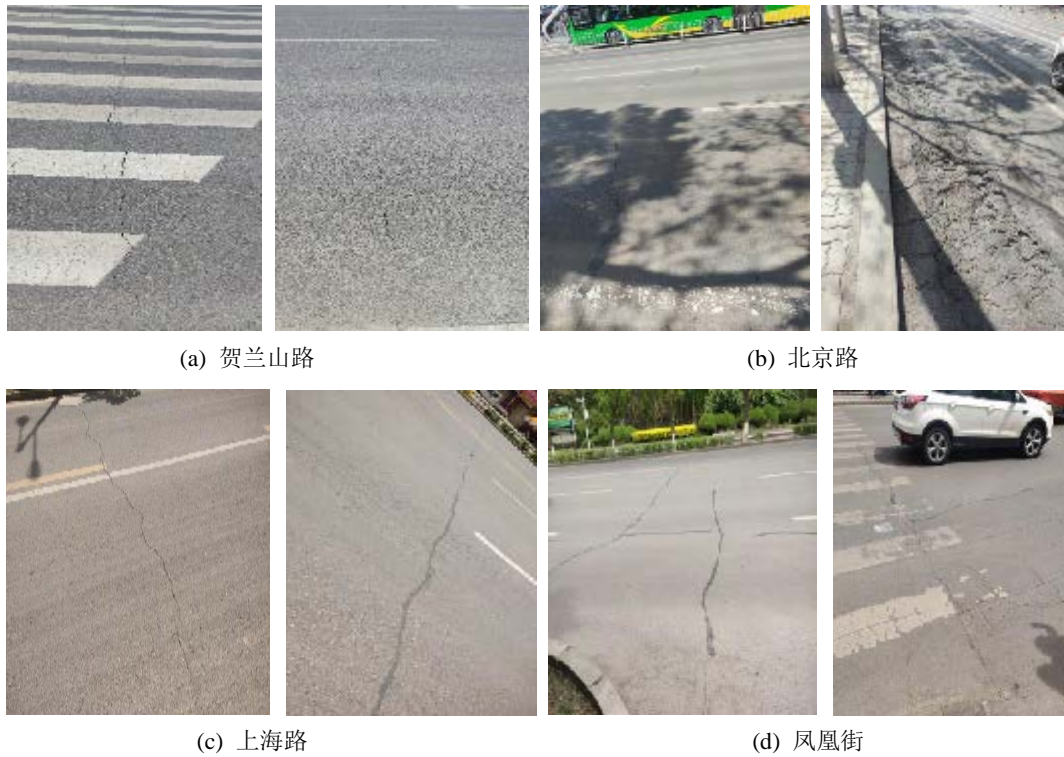
Figure 1. Typical section of pavement damage in Yinchuan 图 1. 银川市典型路段病害情况
