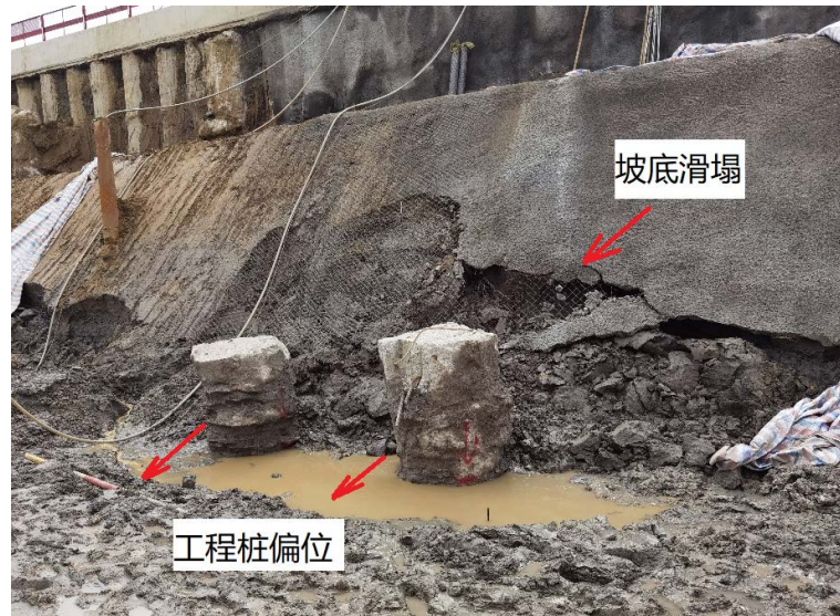
Figure 2. The photo of local collapse of the earth berm 图 2. 反压土坡坡底滑塌照片
