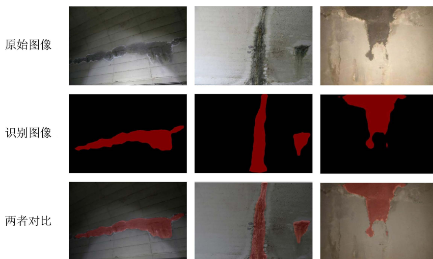
Figure 4. Water leakage identification results 图 4. 渗漏水识别结果
